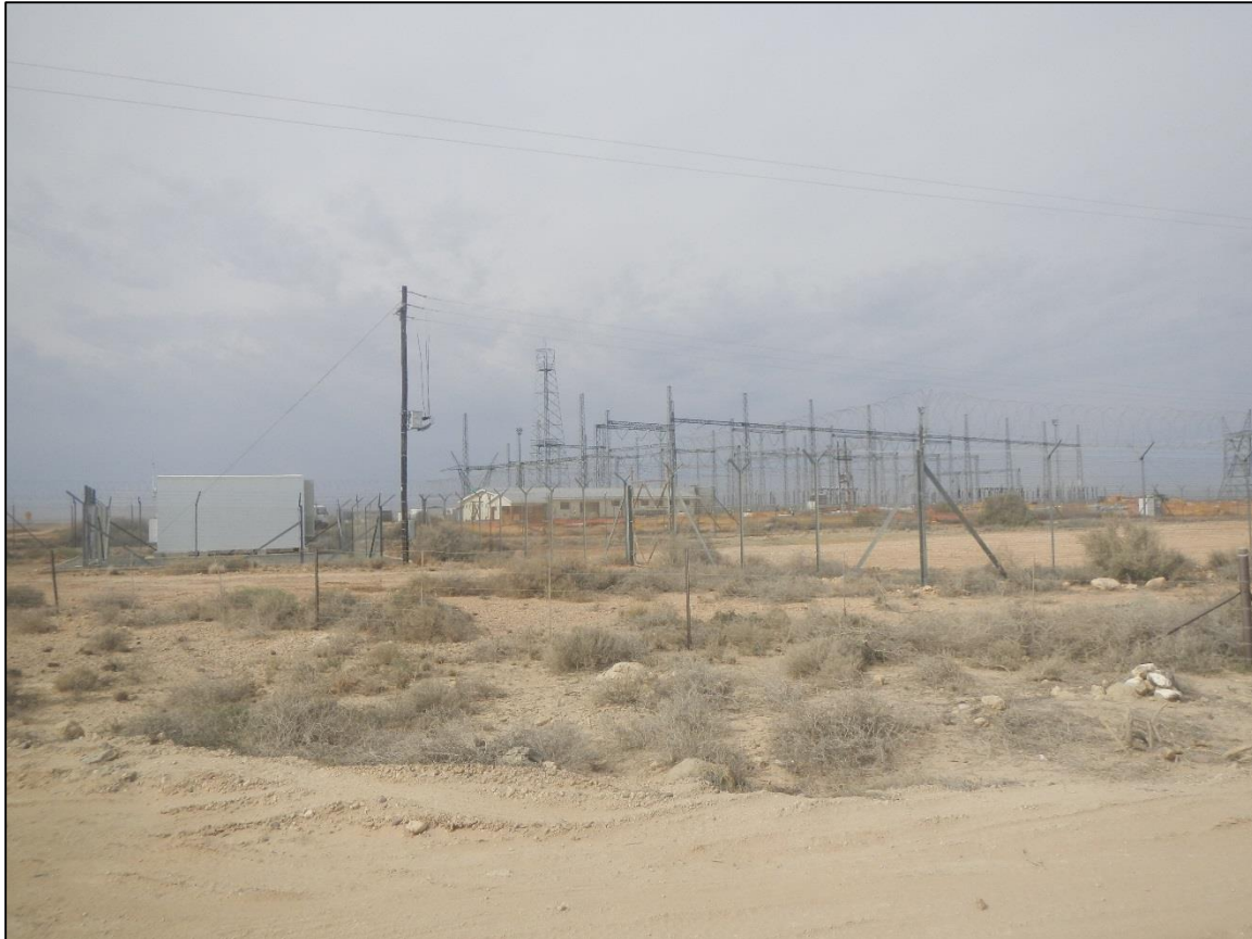
Figure 51: View of the existing Eskom Kronos Substation
