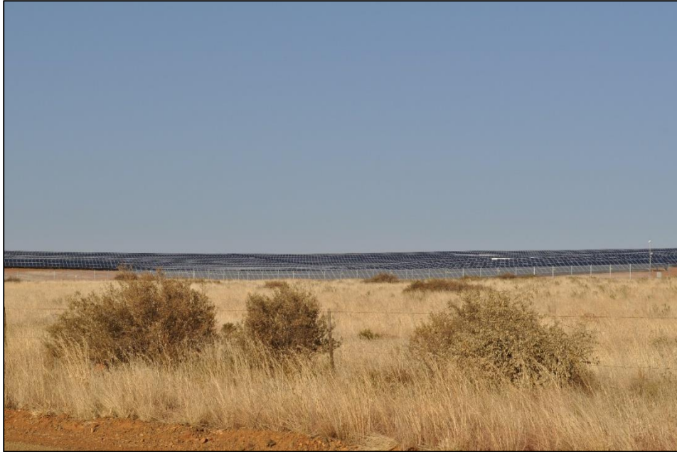
Figure 44: Photovoltaic Panels being erected near Lime Acres in the Northern Cape Province
