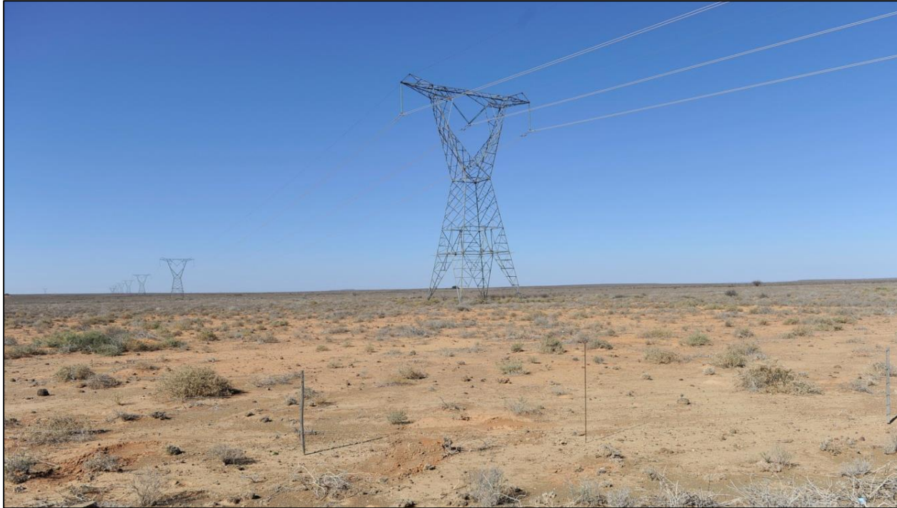
Figure 18: The existing Aries-Kronos 400kV transmission line which runs directly north of the proposed development site.
