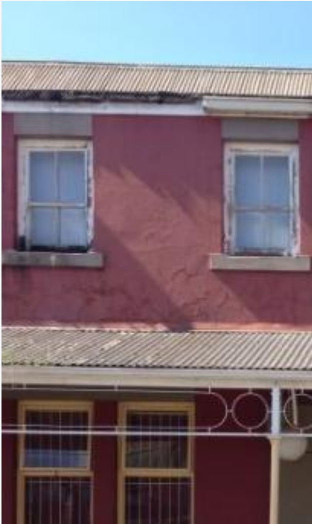
photo 4 Cracking to plaster finish – northwest elevation
