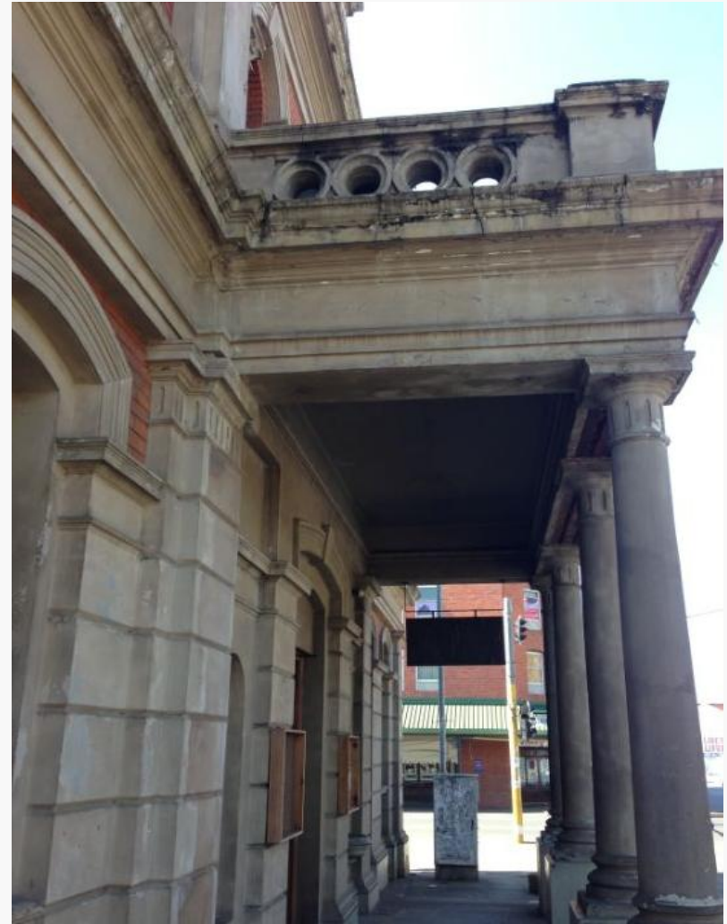
Photo 8 significant cracking to the cornice of the entablature; general poor maintenance and a lack of cleaning evident
