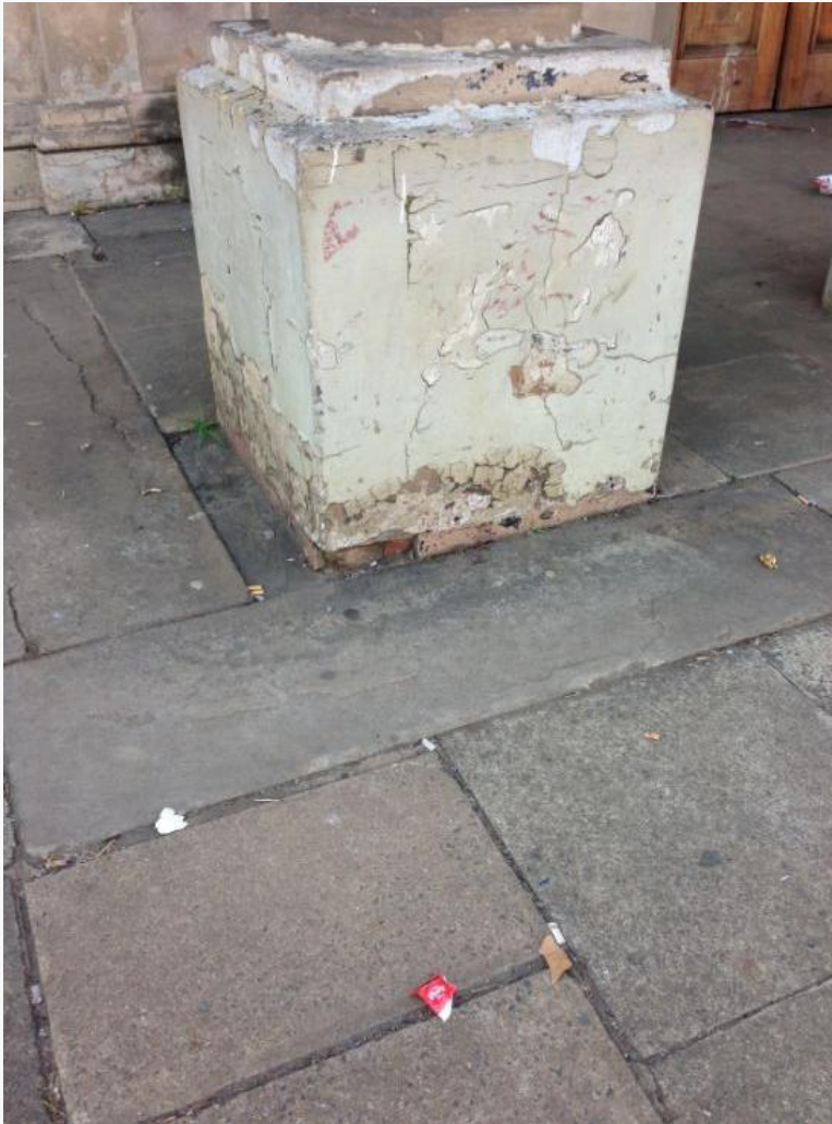
photo 7 Base of column plinth damaged; resultant decay of structure evident
