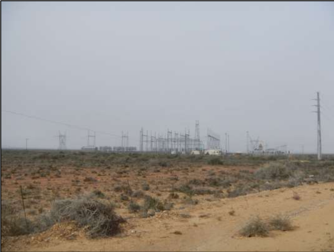
Figure 103: View of the existing Kronos Substation which can be found along the south-western gravel section of the R357 road
