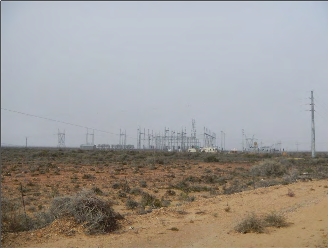
Figure 103: View of the existing Kronos Substation which can be found along the south-western gravel section of the R357 road
