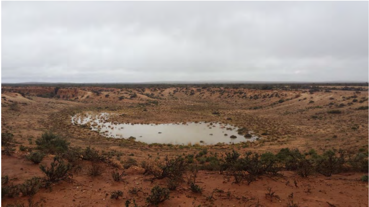
Figure 89: Eroded Edges of an Excavation Pit
