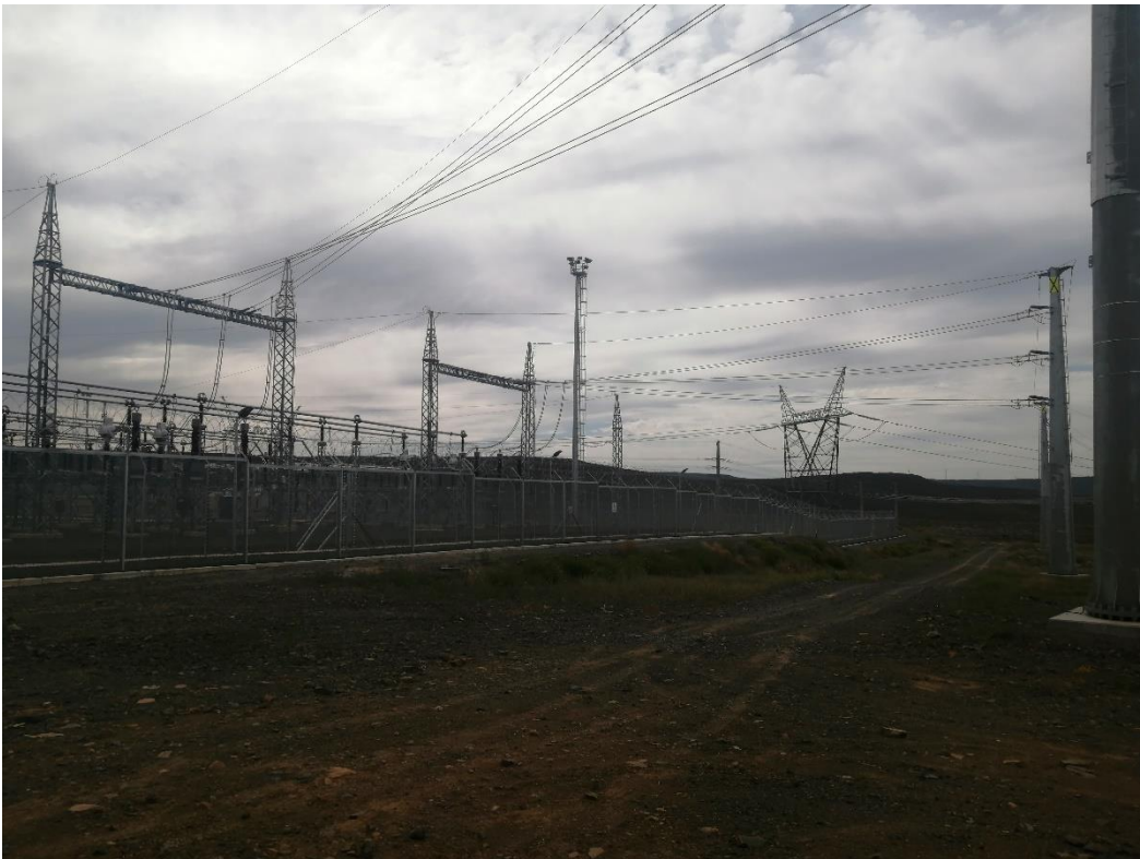
Figure 8: View of the Karusa overhead powerline connection to the Eskom Komsberg substation.
