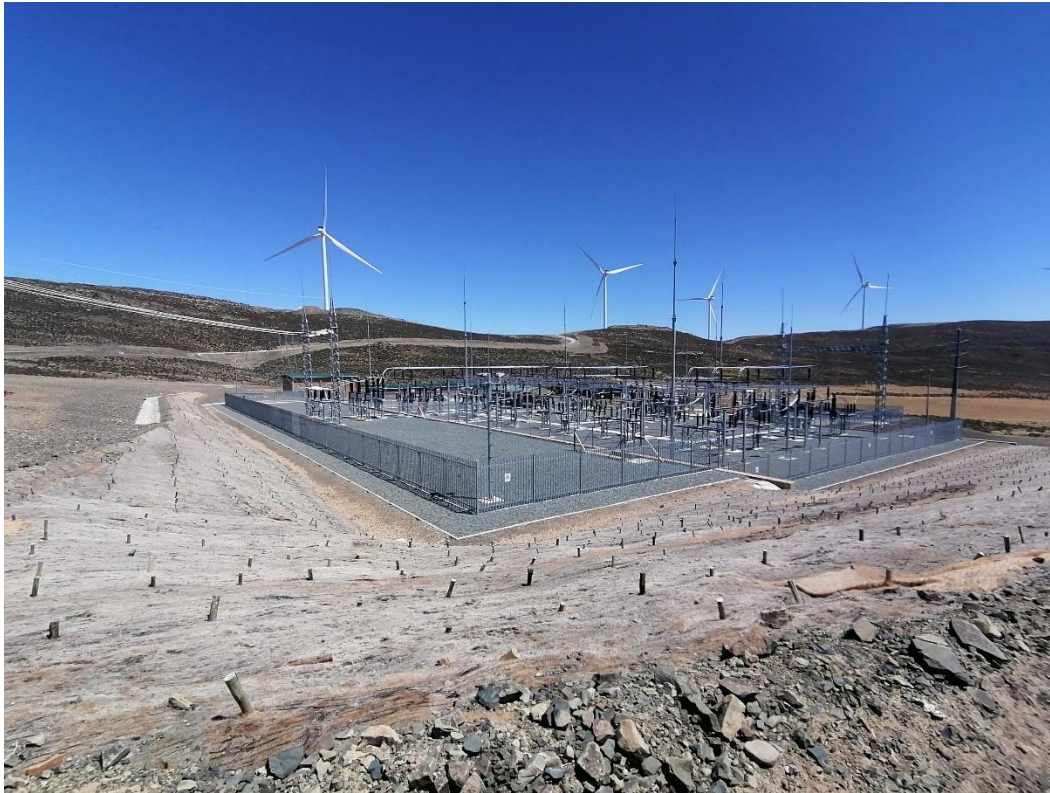
Figure 3: View of the Karusa substation.
