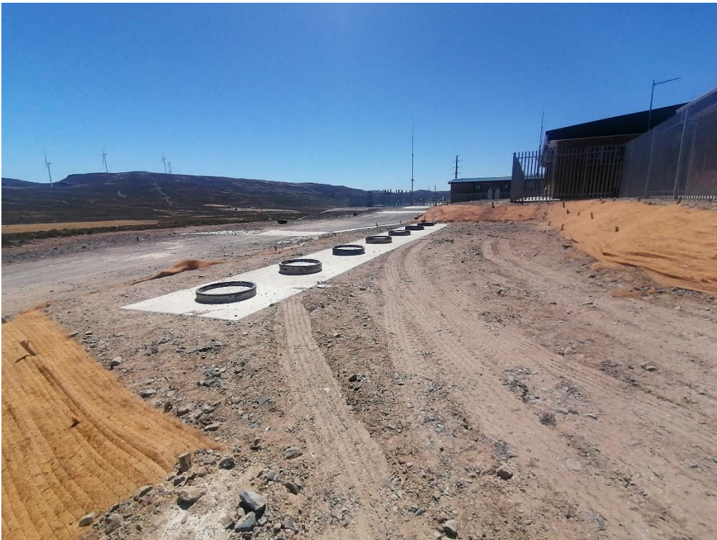
Figure 8: View of conservancy tanks at the Karusa Substation.
