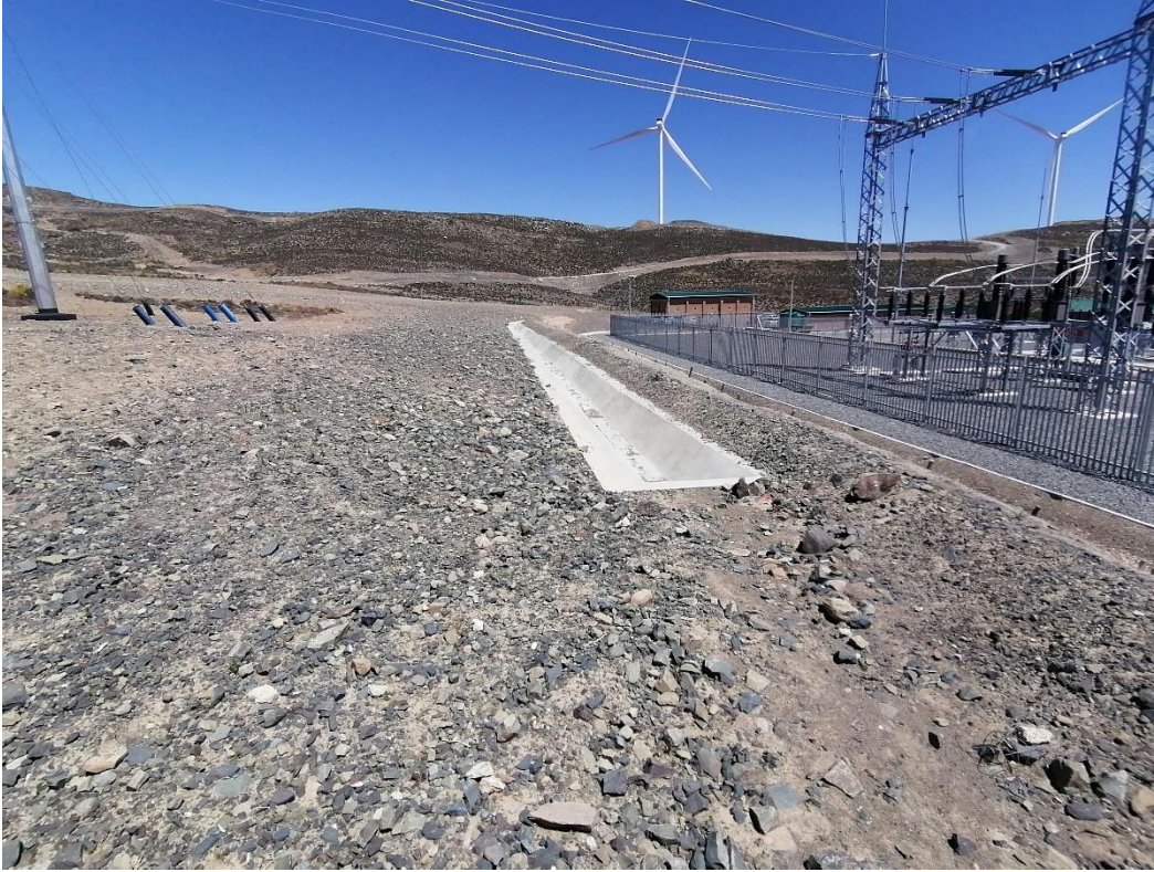
Figure 5: View of stormwater diversion drains along the southern side of the Substation.
