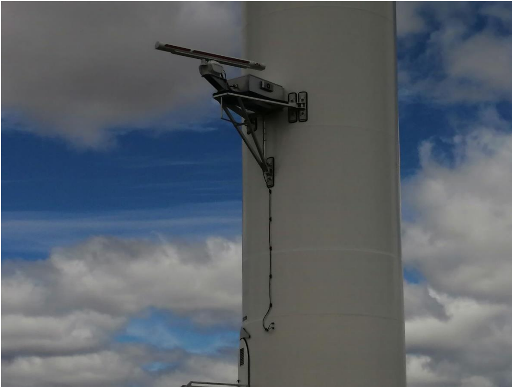
Figure 11: Aircraft Detection Lighting System used on the wind turbines.
