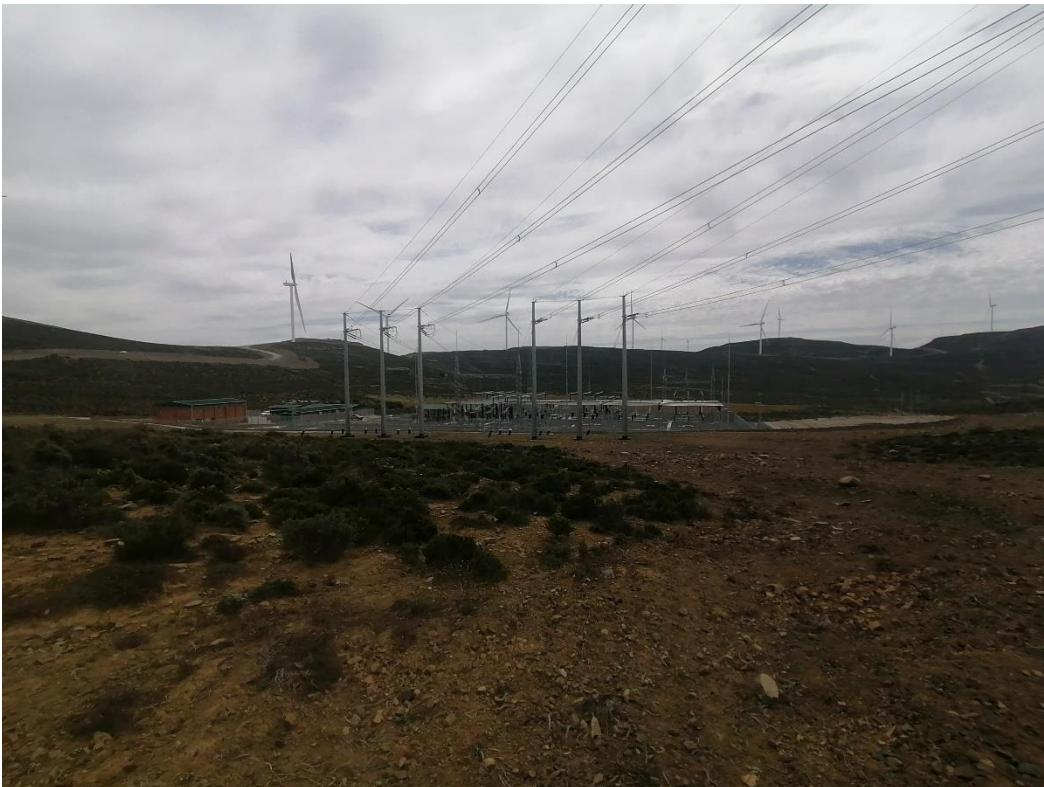
Figure 8: View of the Karusa substation where the Soetwater powerline connects.
