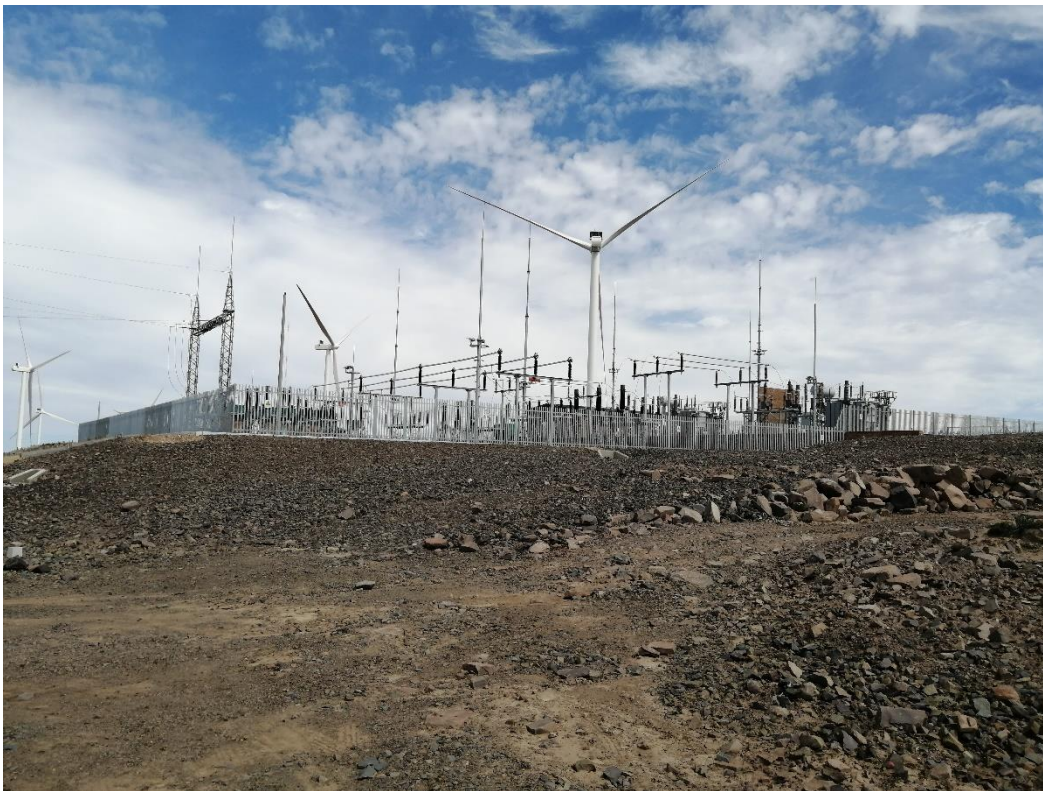
Figure 4: View of the Soetwater substation.
