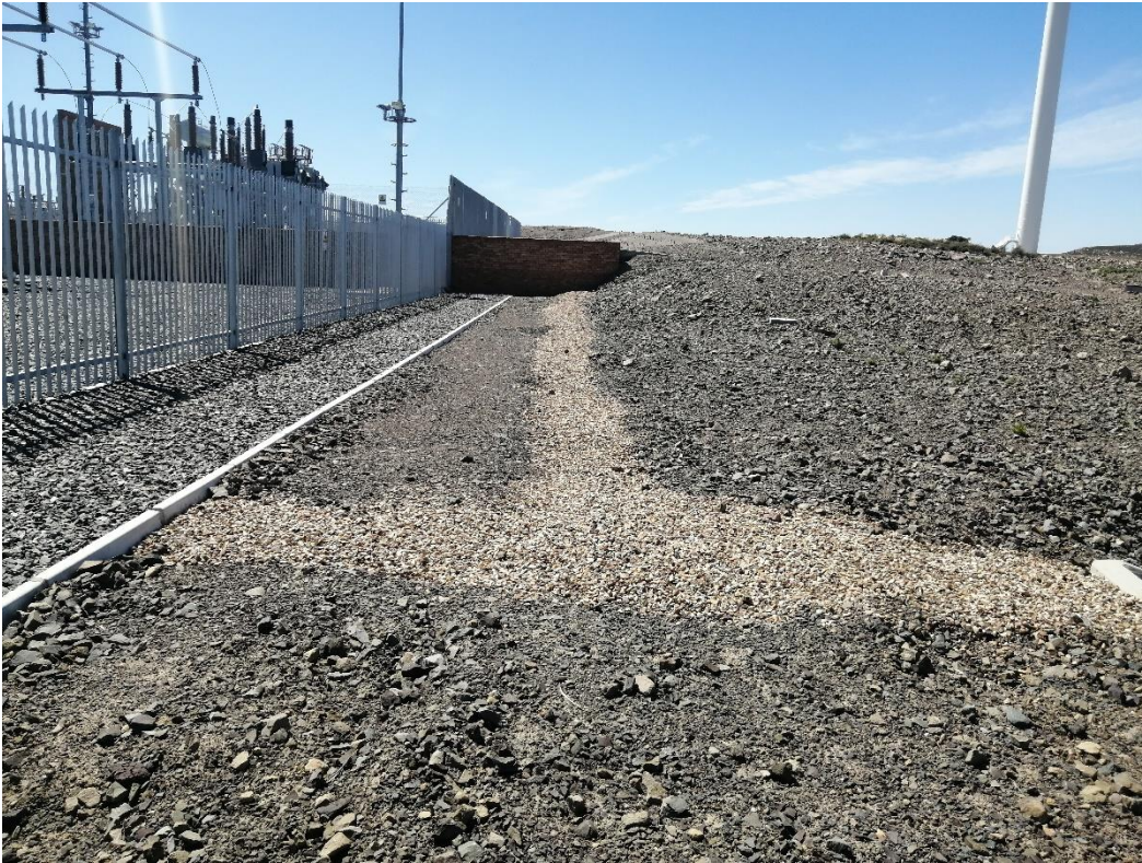
Figure 5: View of subsurface stormwater drains along the northern side of the substation.
