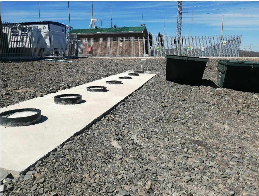
Figure 8: View of conservancy tanks at the Soetwater Substation.
