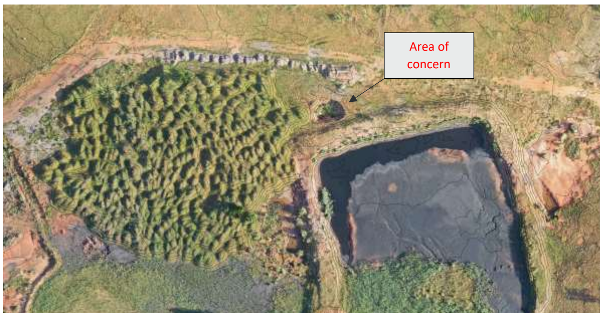
Figure 65: Potential sinkhole formation north of old slurry ponds.
