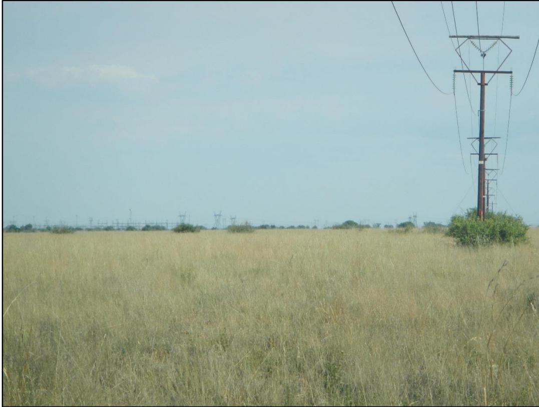
Figure 43: The tall steel structures of the Watershed MTS which can be seen from certain parts of the Lichtenburg Game Breeding Centre.
