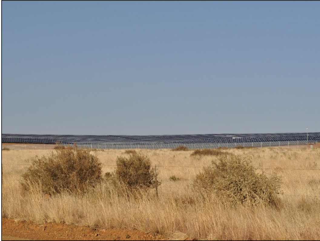
Figure 47: Photovoltaic Panels being erected near Lime Acres in the Northern Cape Province
