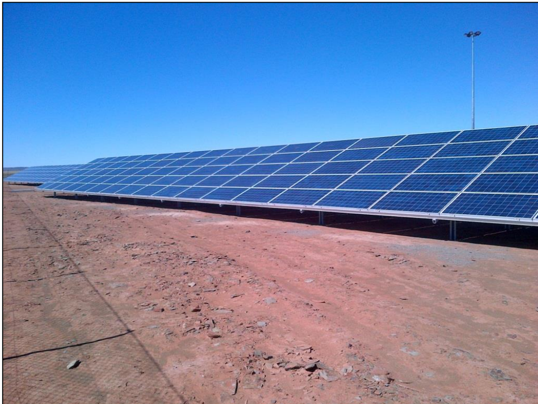
Figure 53: Photovoltaic Panels being erected near De Aar in the Northern Cape Province
