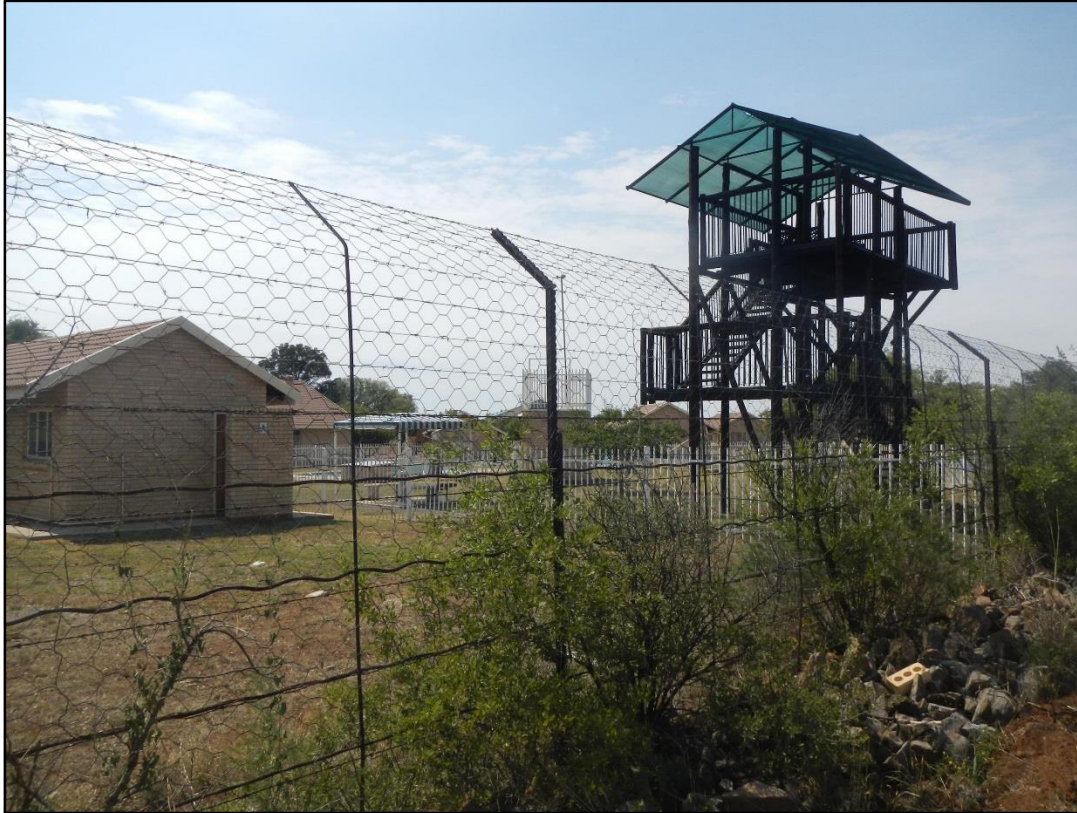
Figure 47: Lookout Tower found in the Lichtenburg Vakansie Oord which looks out over the adjacent Lichtenburg Game Breeding Centre
