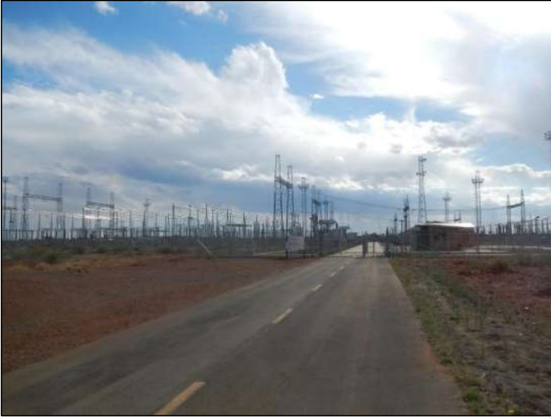
Figure 14: Eskom's newly constructed Mookodi Main Transmission Substation (MTS) which is located to the north-east of the application site
