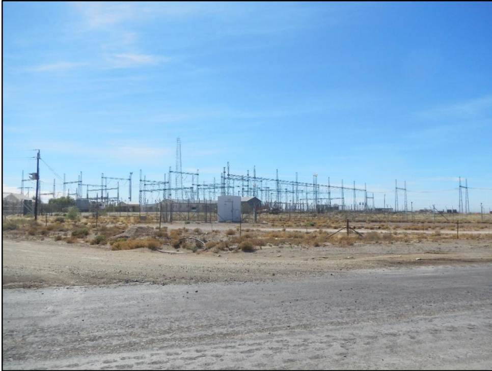
Figure 14: View of the Helios MTS
