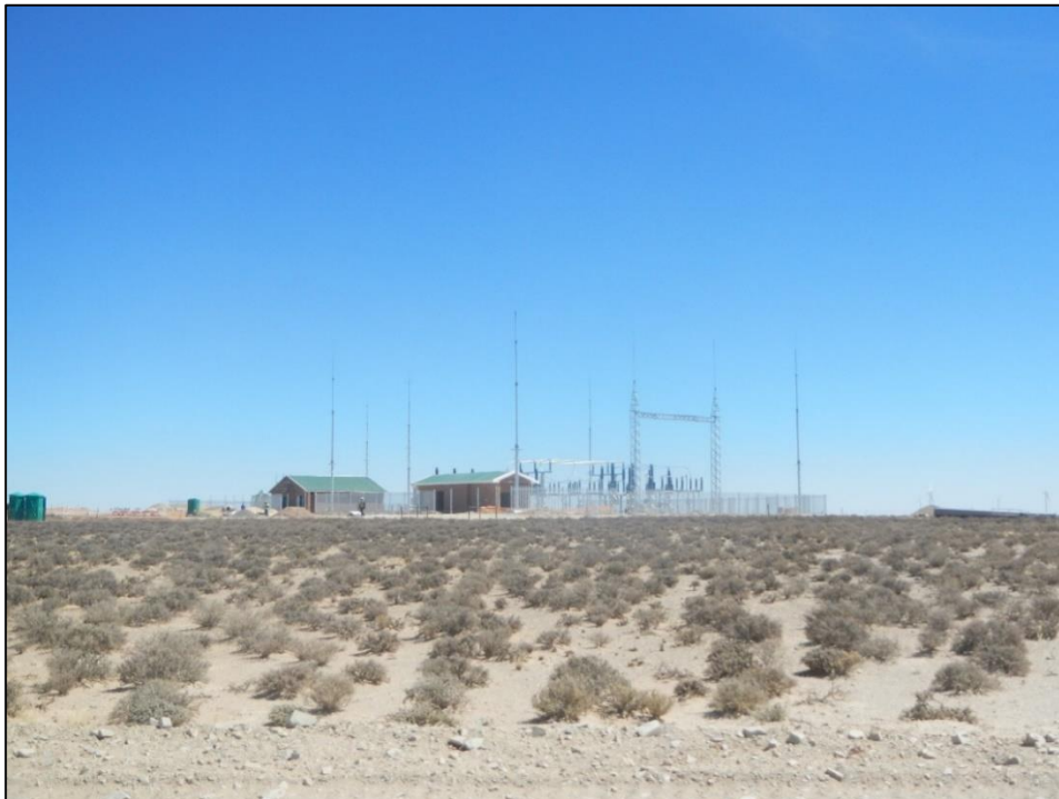
Figure 17: View of the on-site Khobab IPP Substation which had already been constructed during the time of the in-field investigation
