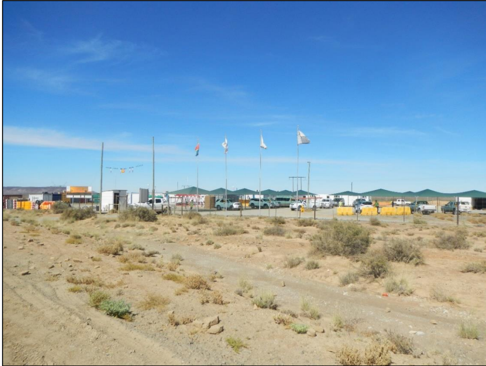
Figure 18: View of the Khobab Wind Farm construction camp area which is situated within the study area, within close proximity to the Helios MTS
