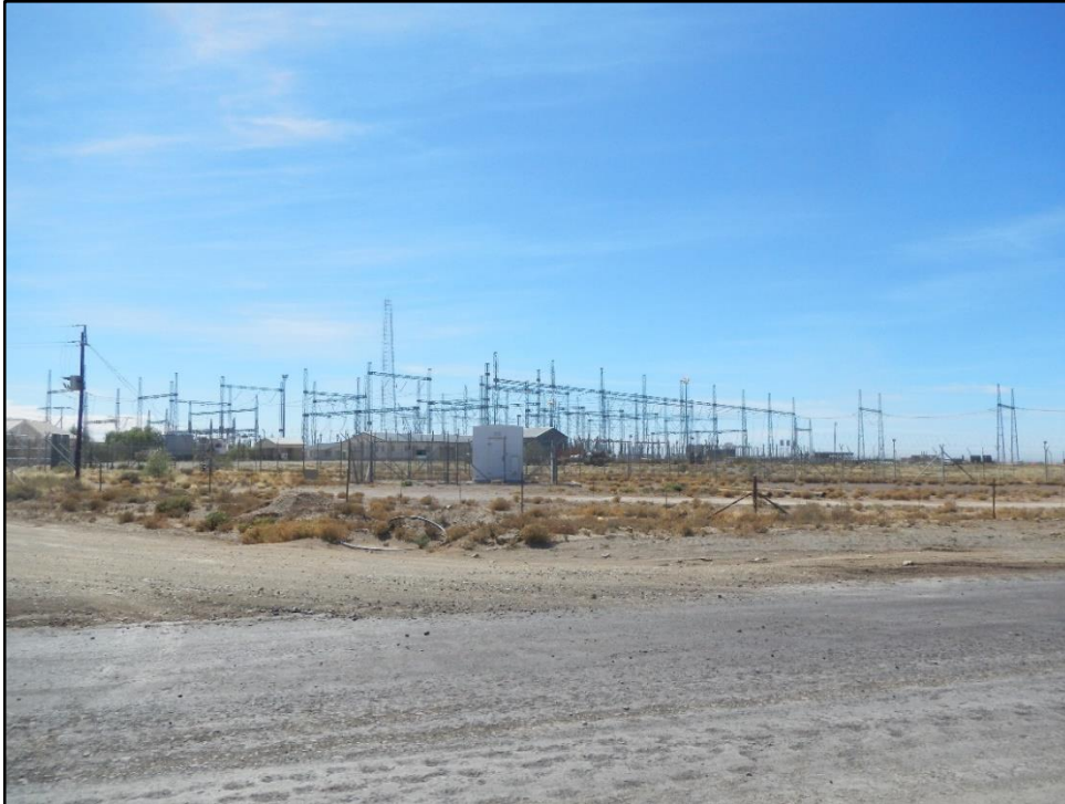
Figure 14: View of the Helios MTS
