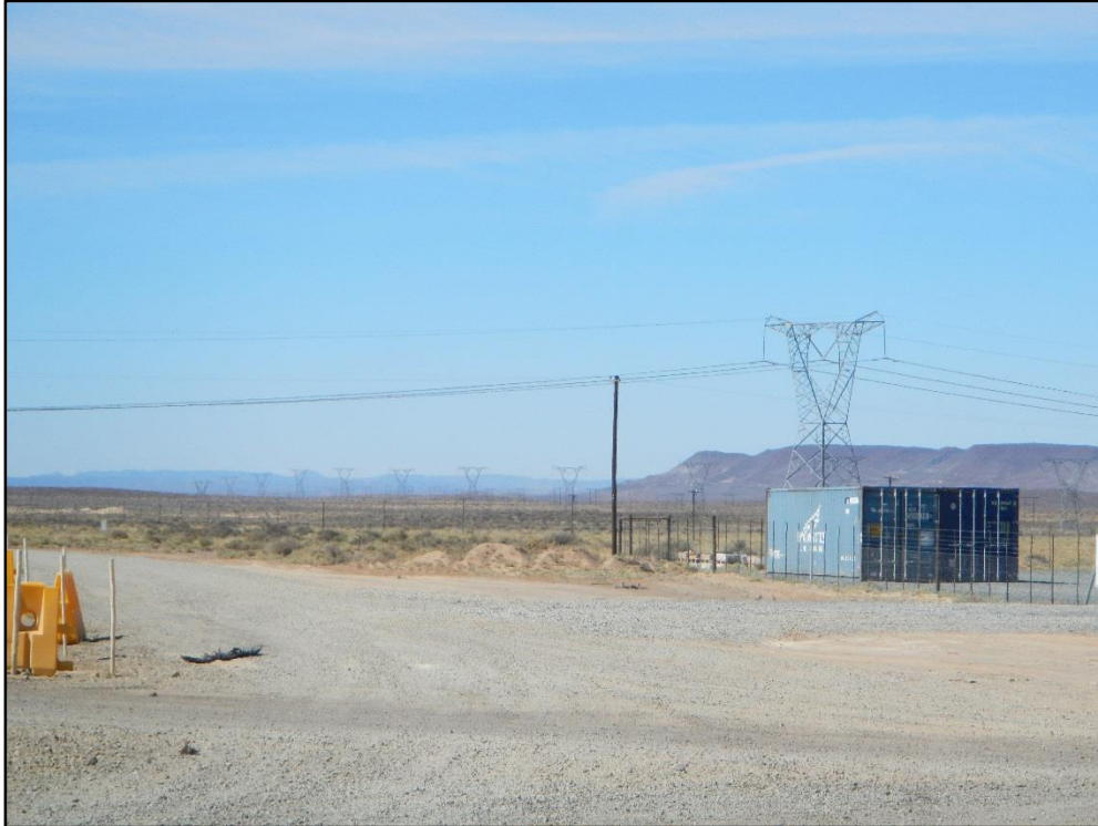
Figure 15: High voltage power lines feeding into Helios MTS
