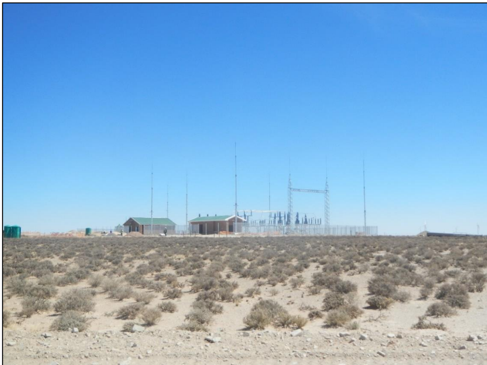
Figure 17: View of the on-site Khobab IPP Substation which had already been constructed during the time of the in-field investigation
