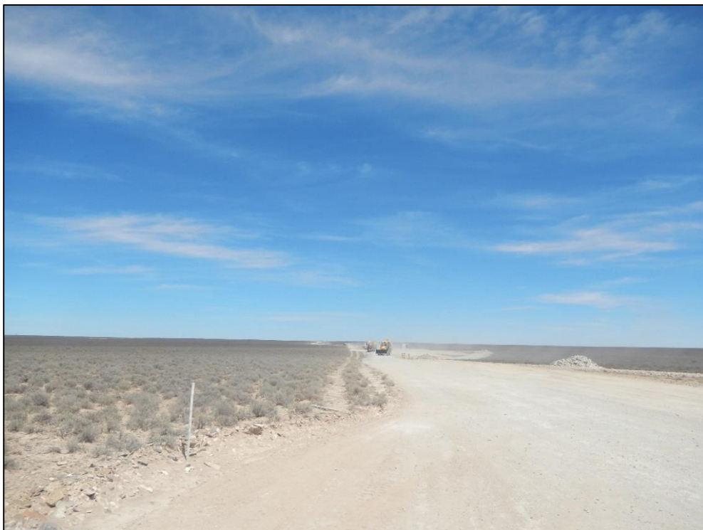
Figure 19: View of the construction activities associated with the proposed Khobab Wind Farm.
