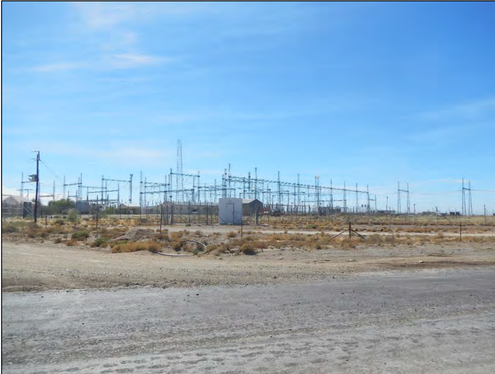
Figure 110: View of the Helios Substation. This substation is however situated well outside of the visual assessment zone
