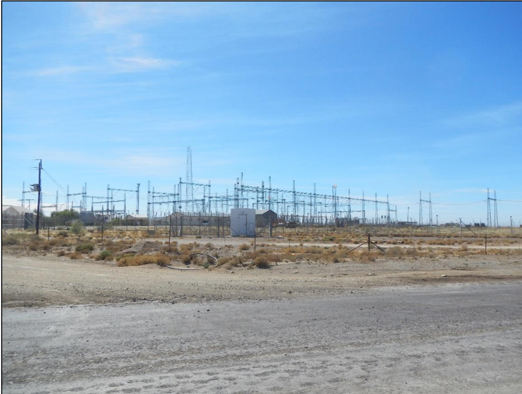
Figure 99: View of the Helios Substation. This substation is however situated well outside of the visual assessment zone
