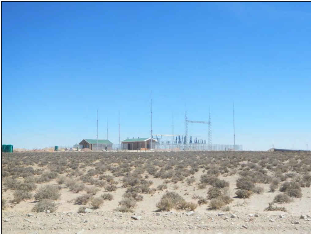
Figure 105: View of the on-site Khobab IPP Substation which had already been constructed during the time of the in-field investigation. This on-site IPP Substation is however located well outside of the visual assessment zone.
