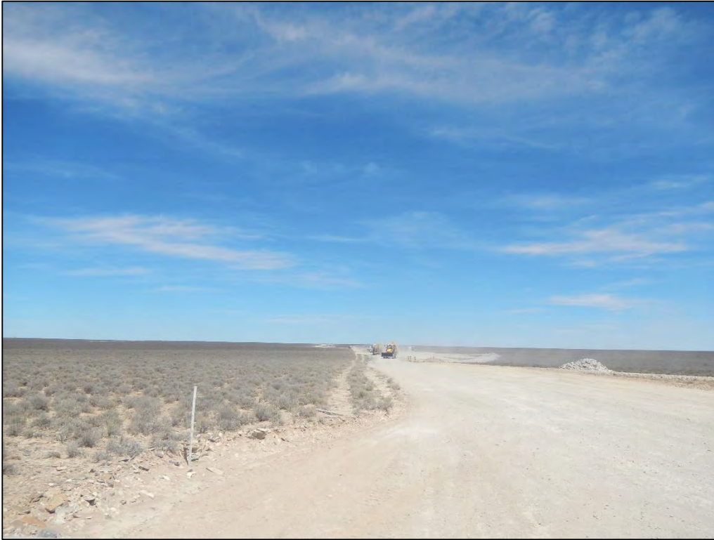
Figure 109: View of the construction activities associated with the proposed Khobab Wind Farm. During the time of the in-field investigation it was noted that this wind farm was still in the early stages of construction and no turbines had thus been erected.
