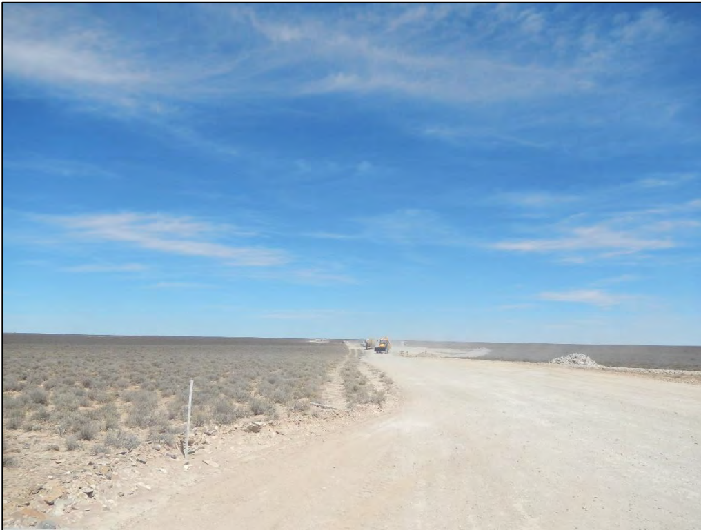
Figure 98: View of the construction activities associated with the proposed Khobab Wind Farm. During the time of the in-field investigation it was noted that this wind farm was still in the early stages of construction and no turbines had thus been erected.
