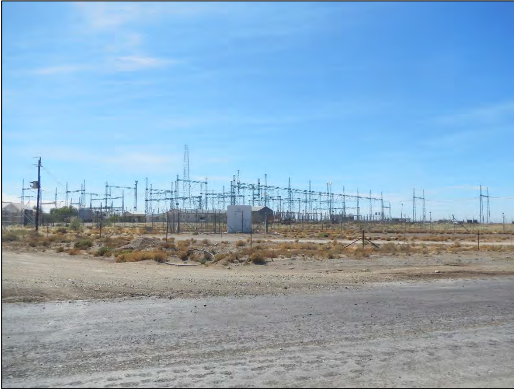
Figure 99: View of the Helios Substation. This substation is however situated well outside of the visual assessment zone
