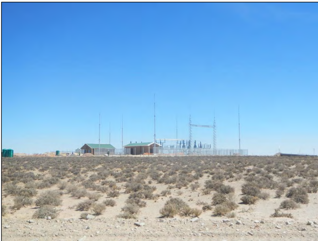
Figure 104: View of the on-site Khobab IPP Substation which had already been constructed during the time of the in-field investigation. This on-site IPP Substation is however located well outside of the visual assessment zone.
