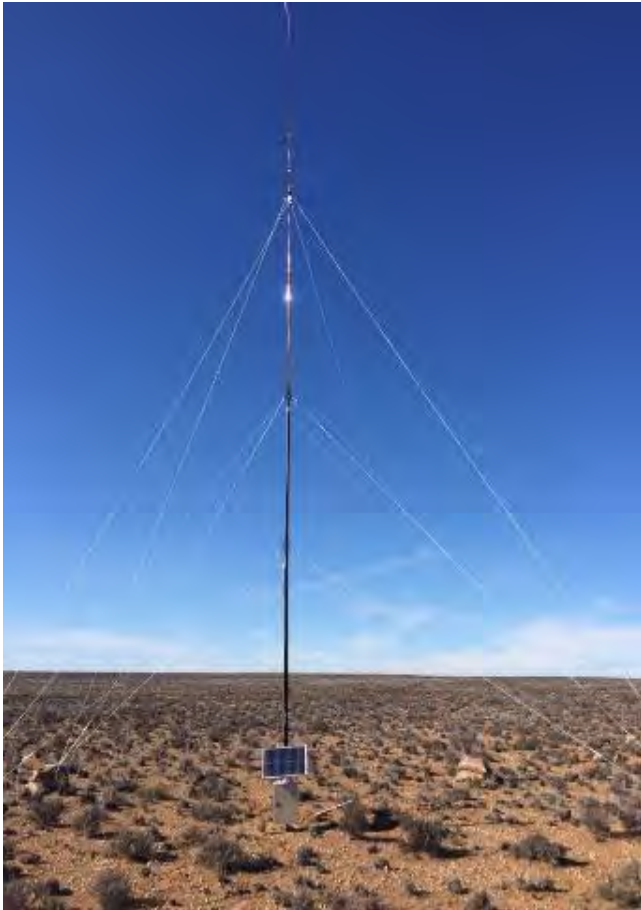
Figure 48: Short mast monitoring system
