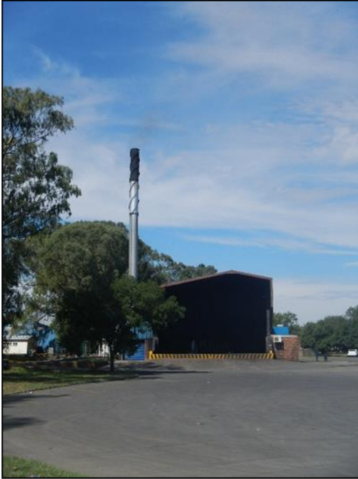
Figure 3: Existing John Thompson 20 bar Boiler at the Kliprivier Mill
