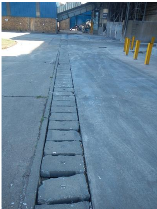
Figure 6: Storm water drainage systems found around various buildings/structures at the Kliprivier Mill
