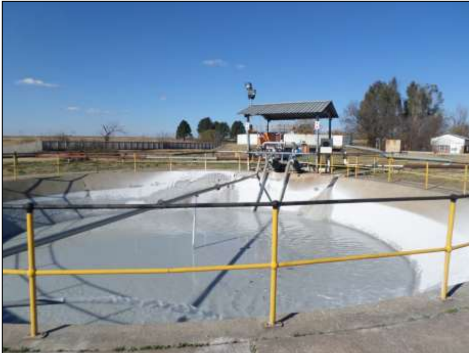
Figure 4: Onsite Effluent Treatment Facility at the Kliprivier Mill
