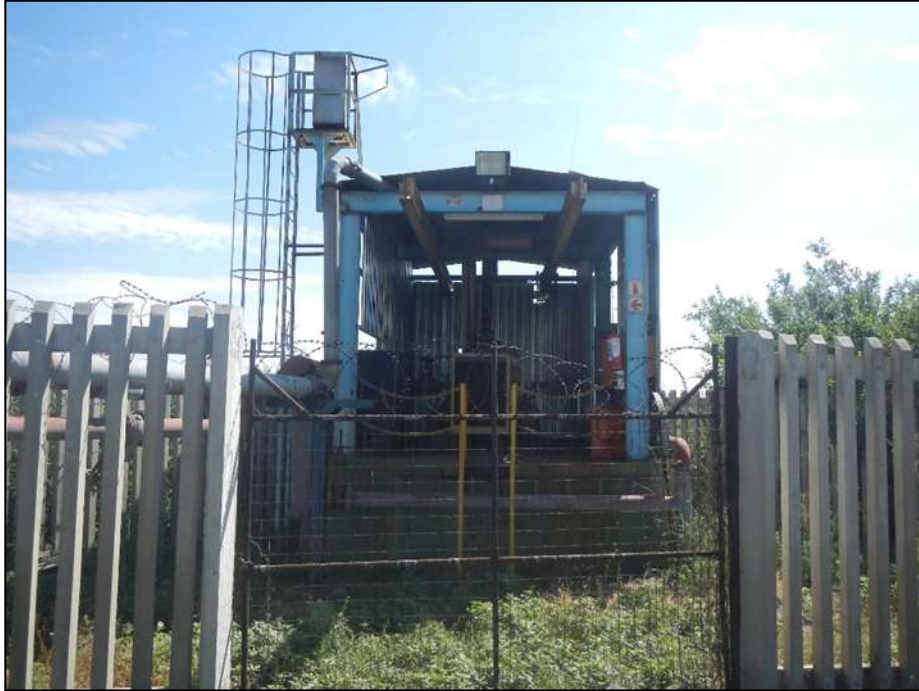
Figure 2: Pump Station found within close proximity to the Kliprivier. Used to draw water from the river in case of fire outbreaks only.
