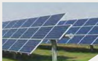
Terraform Portfolio OE - 110MW AC Portfolio of 3 projects, Boshof, Witkop and Soutpan
