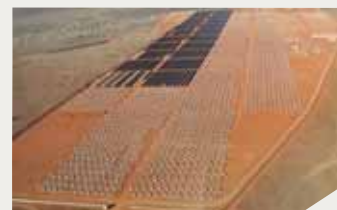
Lesedi PV Installation
