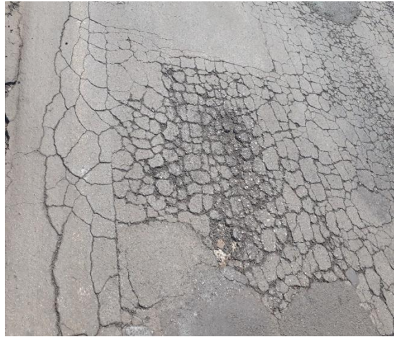
Photograph 3.4: Crocodile cracks in the pavement
