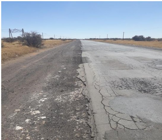
Photograph 3.5: non-existing road edge
