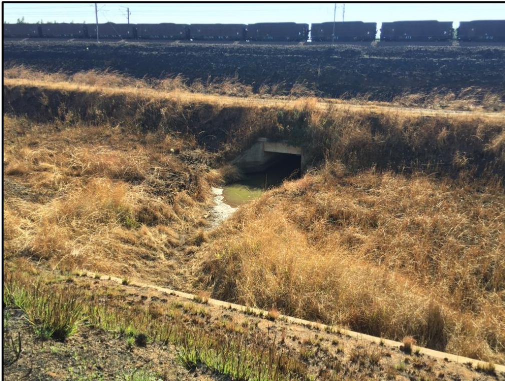
Photo 4: Stormwater drainage / culvert crossed over, which is small and typical of all of those found in the study area
