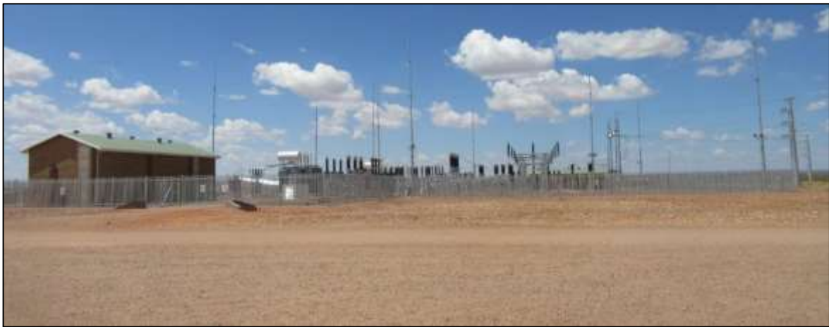
Photograph 3.11: Dyasonsklip 1 and SEF substation and 132 kV line just to the south of the Dyasonsklip 5 site
