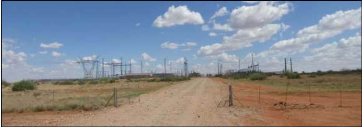
Photograph 3.9: Eskom's Upington MTS substation
