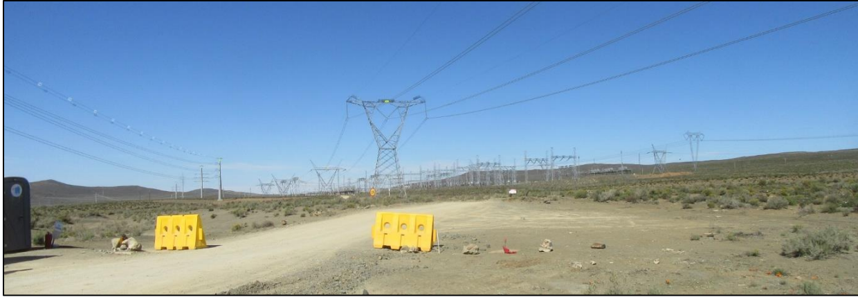
Photograph 3.11: Eskom's Komsberg substation, viewed from the entrance along the Komsberg Road
