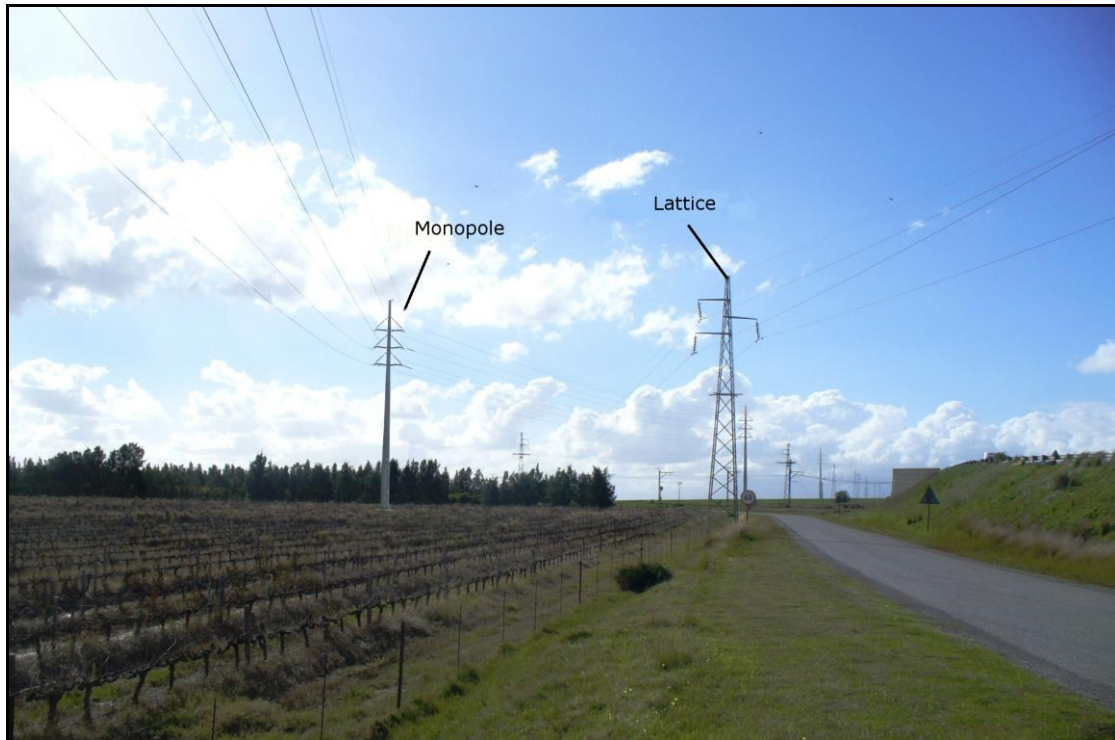
Figure 3: Longer distance view of power line towers.
