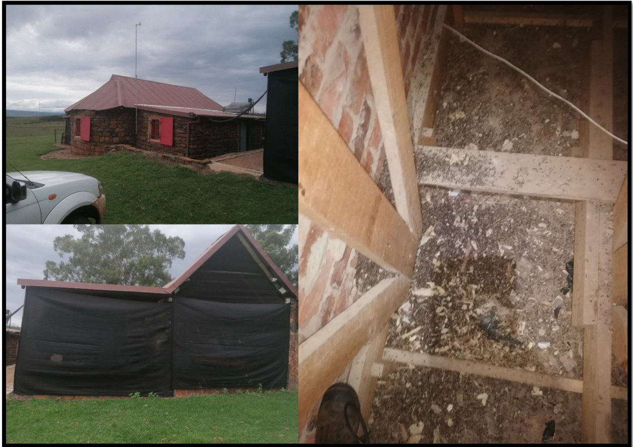
Figure 33. Examples of potential roosts with evidence of bats on the right
