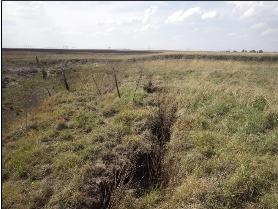
Figure 7-6: Fractures in the banks of the Rietspruit at MAT5 (October 2016)
