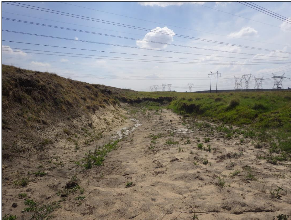
Figure 7-7: Erosion and sedimentation observed at BP1 during the low flow survey
