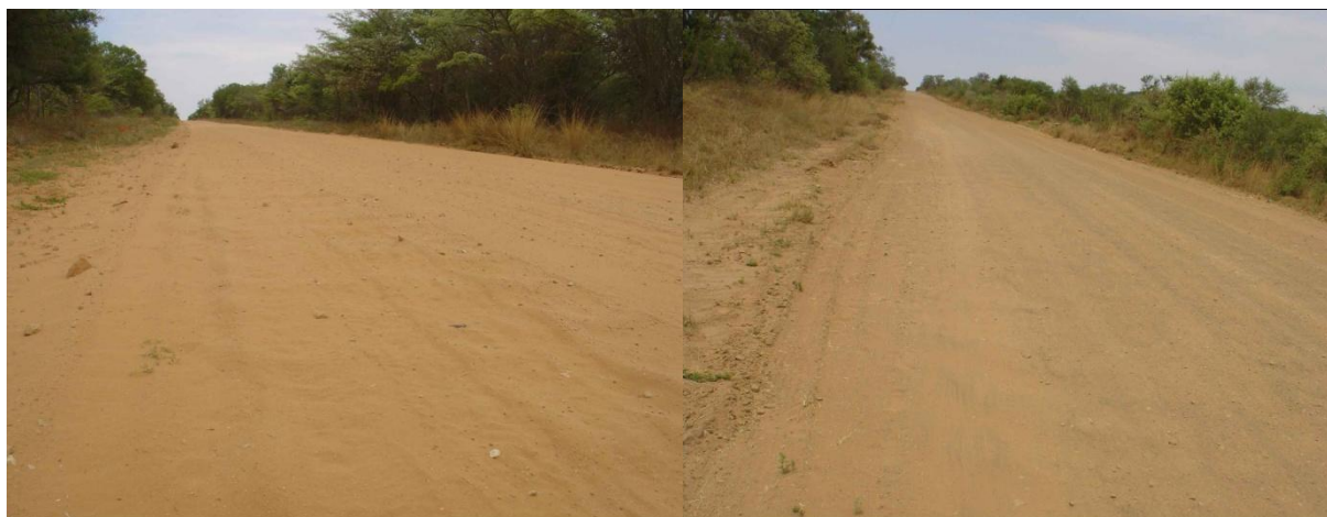
Photo 3 – Silt on Road D2747
