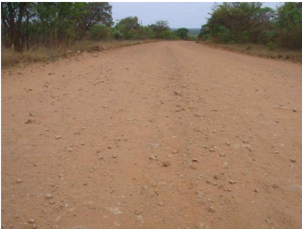
Photo 1 – Gravel on Road D2747
