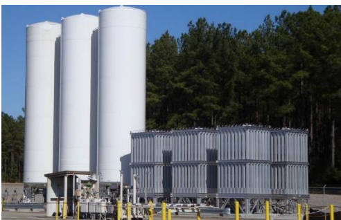
Figure 9: Typical vertical LNG cryogenic bulk storage tanks. A single 300m 3 storage tank typically stores 145 tonnes of LNG.
