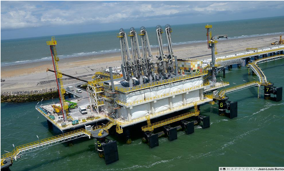
Figure 4: LNG vessel docking/ mooring station complete with LNG cryogenic unloading mechanisms located on the LNG Terminal.
