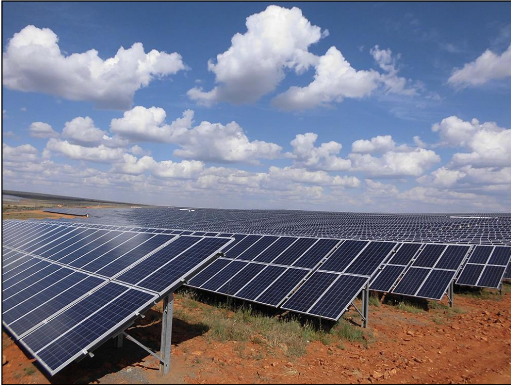
Figure 6-5: The Lesedi PV Project near Kimberley in the Northern Cape 7 .
