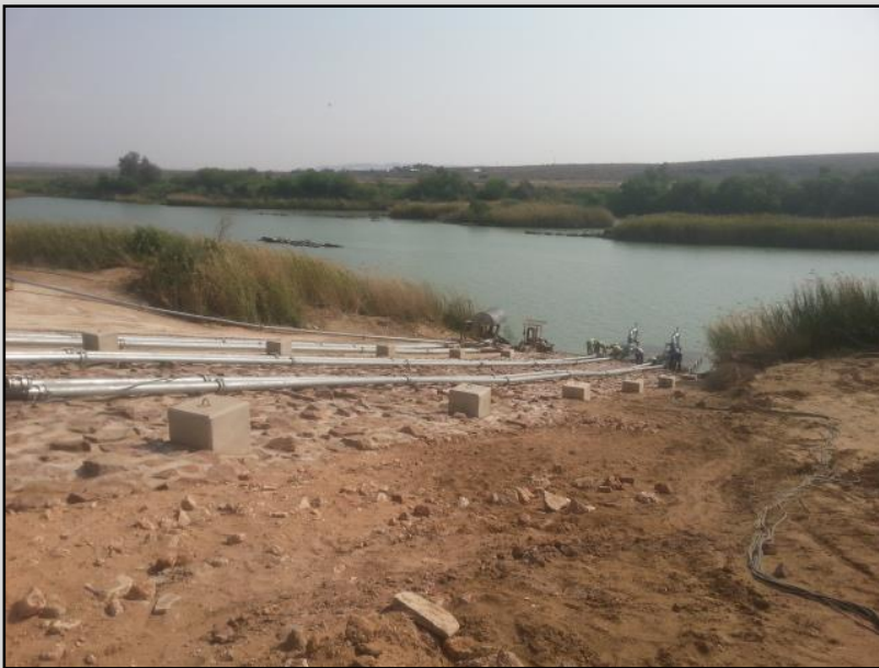
View of the approximate area for the construction of the abstraction point (Bokpoort I abstraction infrastructure is shown in the photo).
