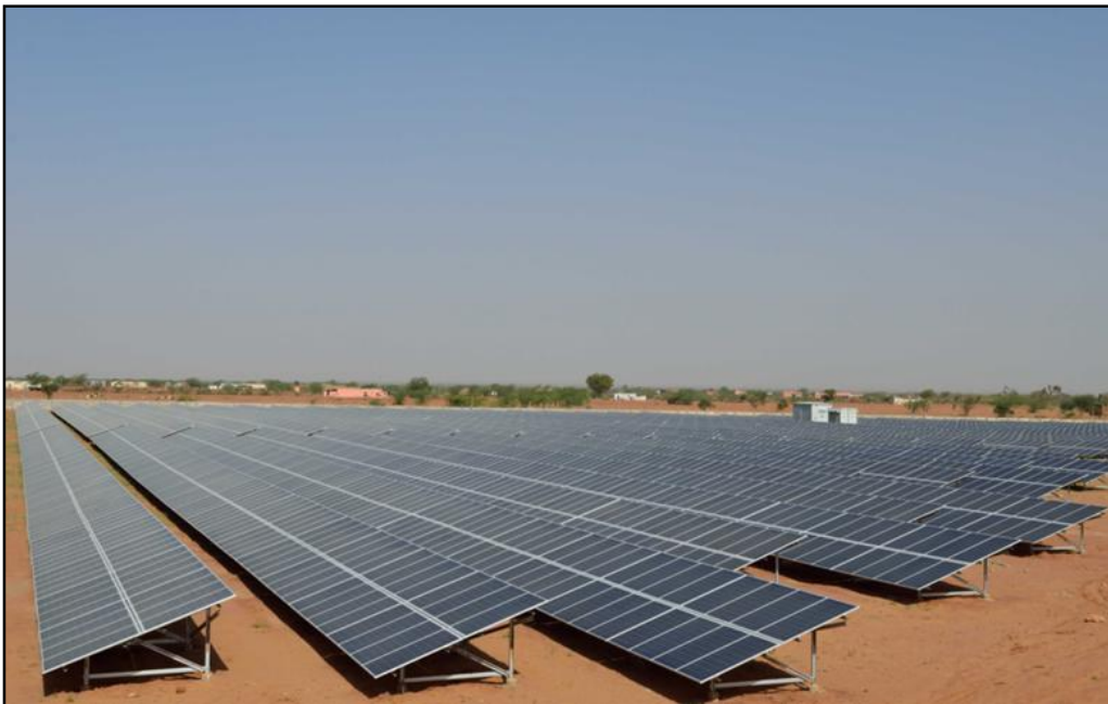
Figure 3-2: Example of PV Solar Power Facility's Tracker View 2
