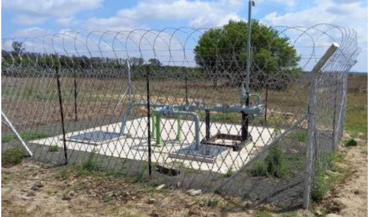
Figure 10: View of an existing pigging station constructed as part of Cluster 1.
