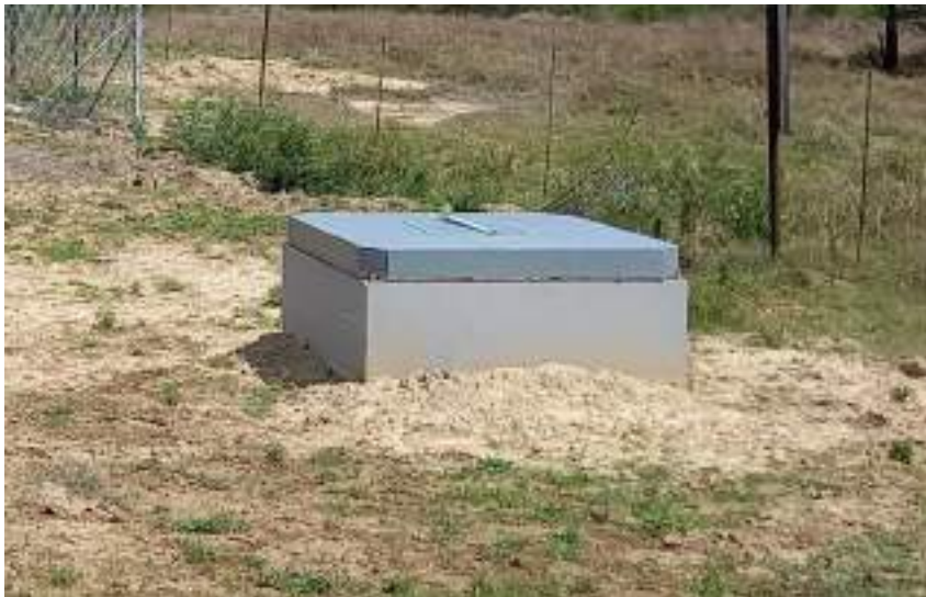
Figure 11: View of an existing low point drain constructed as part of Cluster 1.
