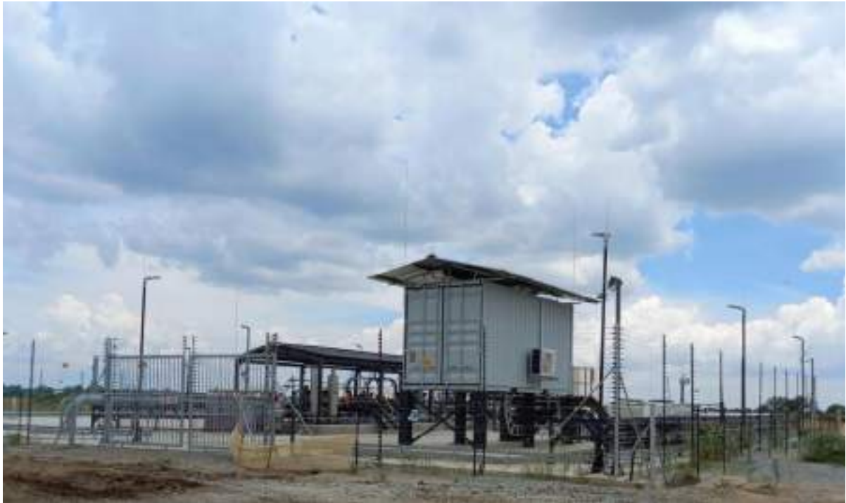
Figure 12: Example of Compressor Station just recently constructed as part of Cluster 1.
