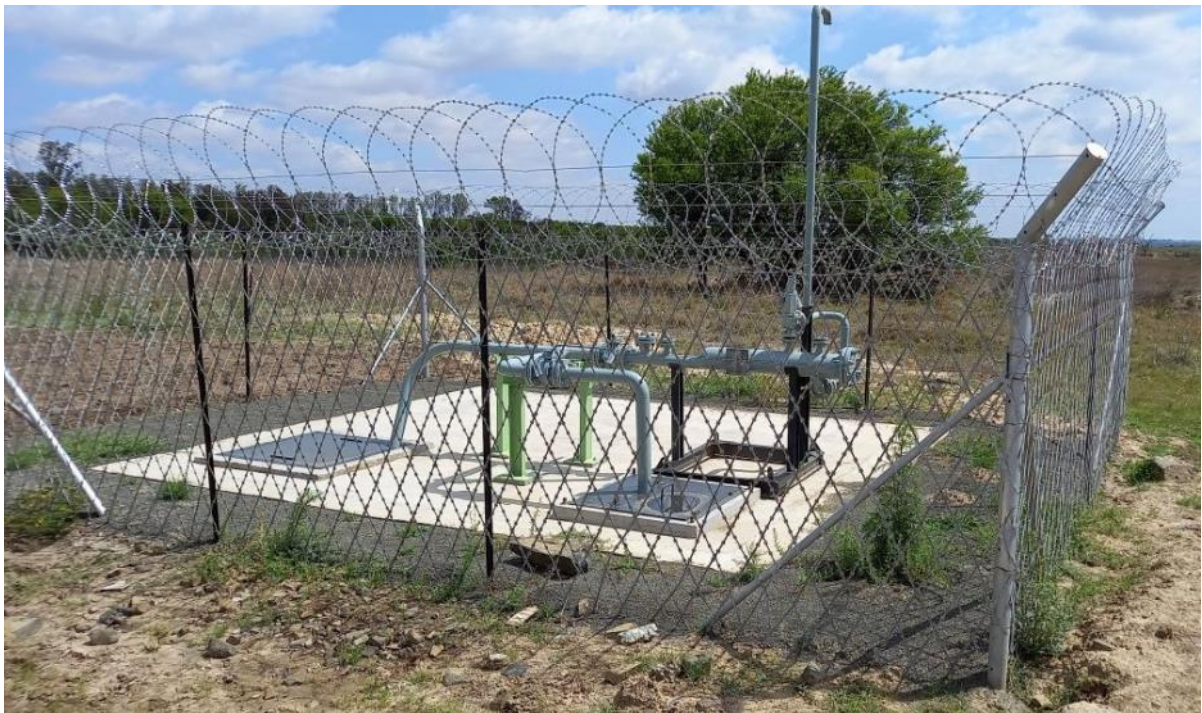
Figure 8: View of an existing pigging station constructed as part of Cluster 1.
