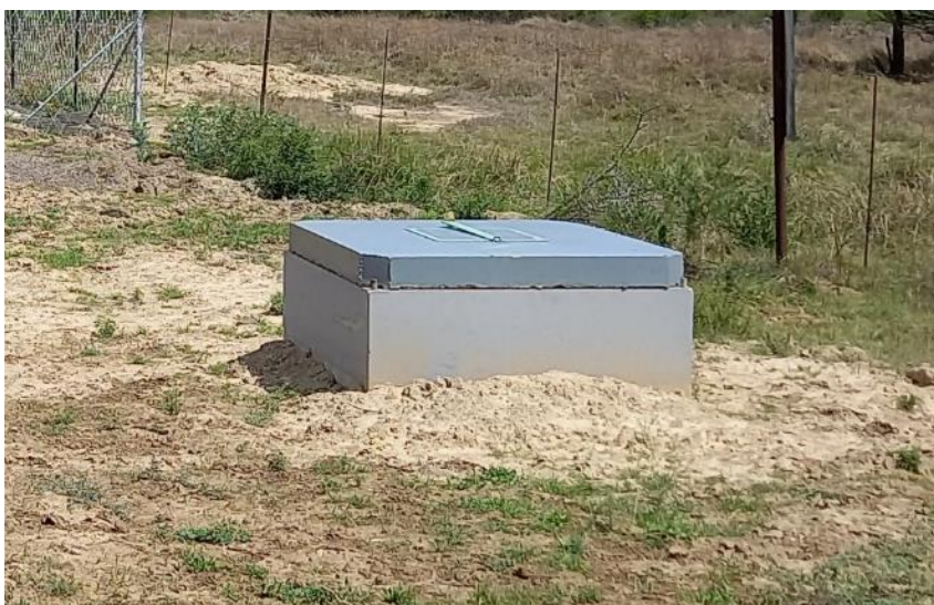
Figure 9: View of an existing low point drain constructed as part of Cluster 1.
