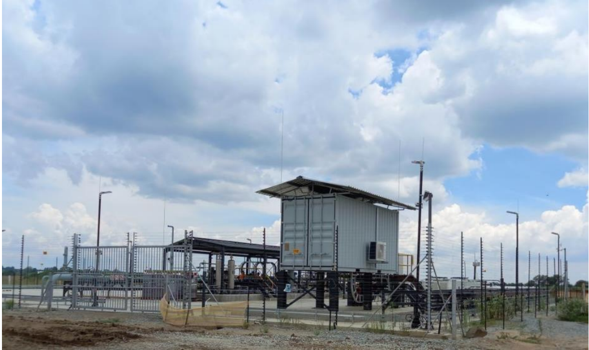
Figure 10: Example of Compressor Station just recently constructed as part of Cluster 1.
