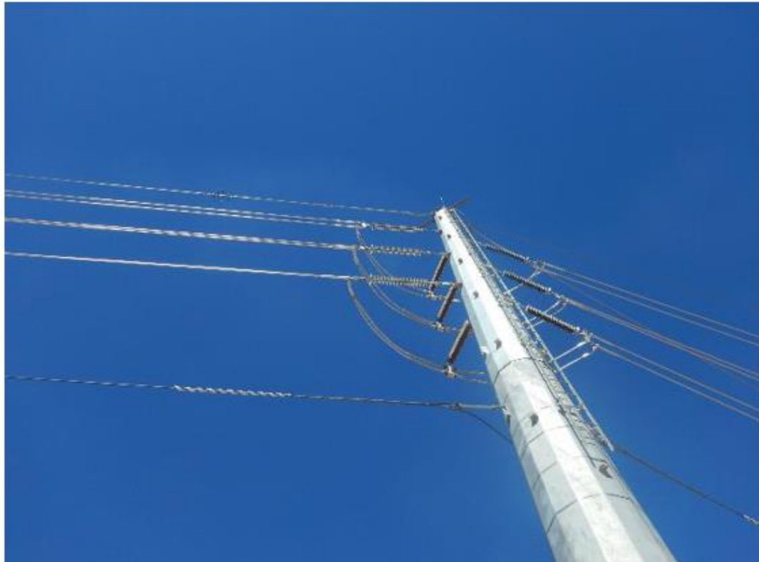
Figure 7: HV Lines: Cuprum bay and terminal structure
