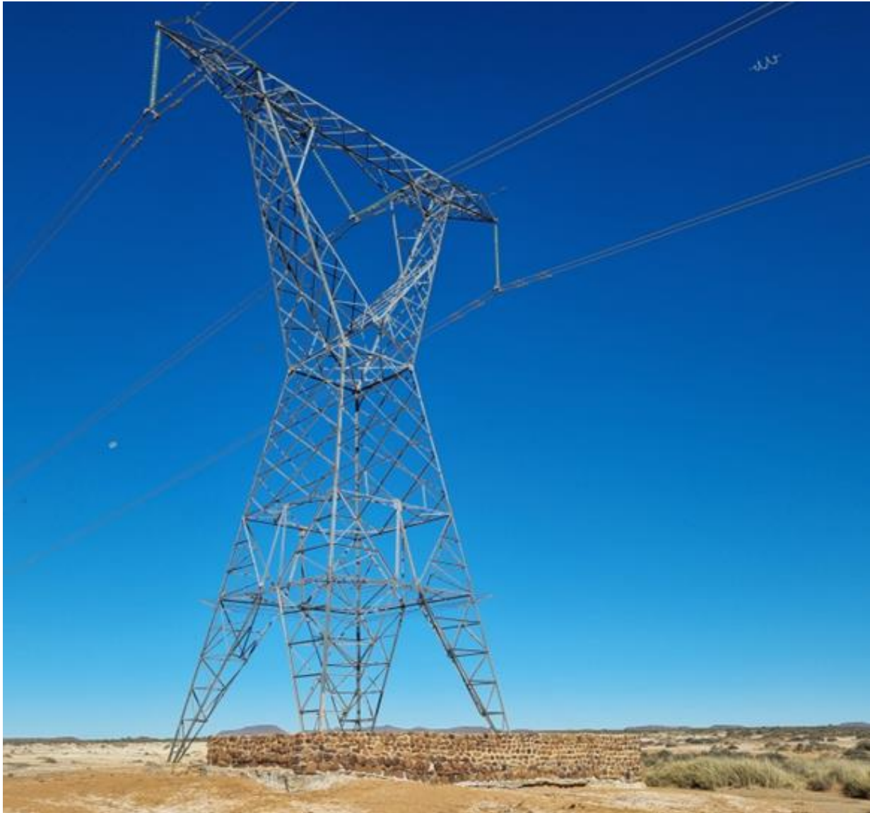
Figure 1-1: Existing transmission line from the Hydra to Kronos Substations
