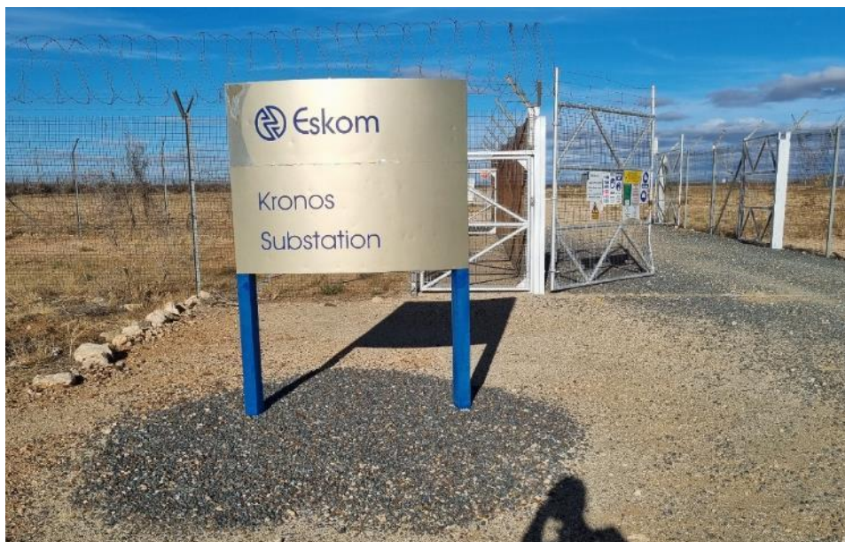
The Kronos Substation which the proposed 400 kV Line will be connected (June 2023)
