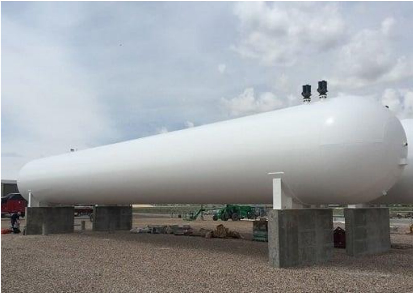
Figure 14: Bullet storage tank (ammonia storage)
