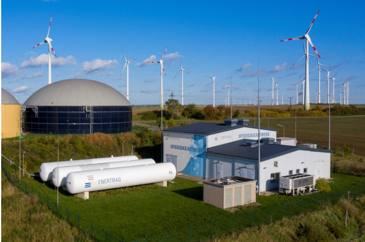
Figure 2: Closer View of Electrolyser Housing and Storage Tanks.
