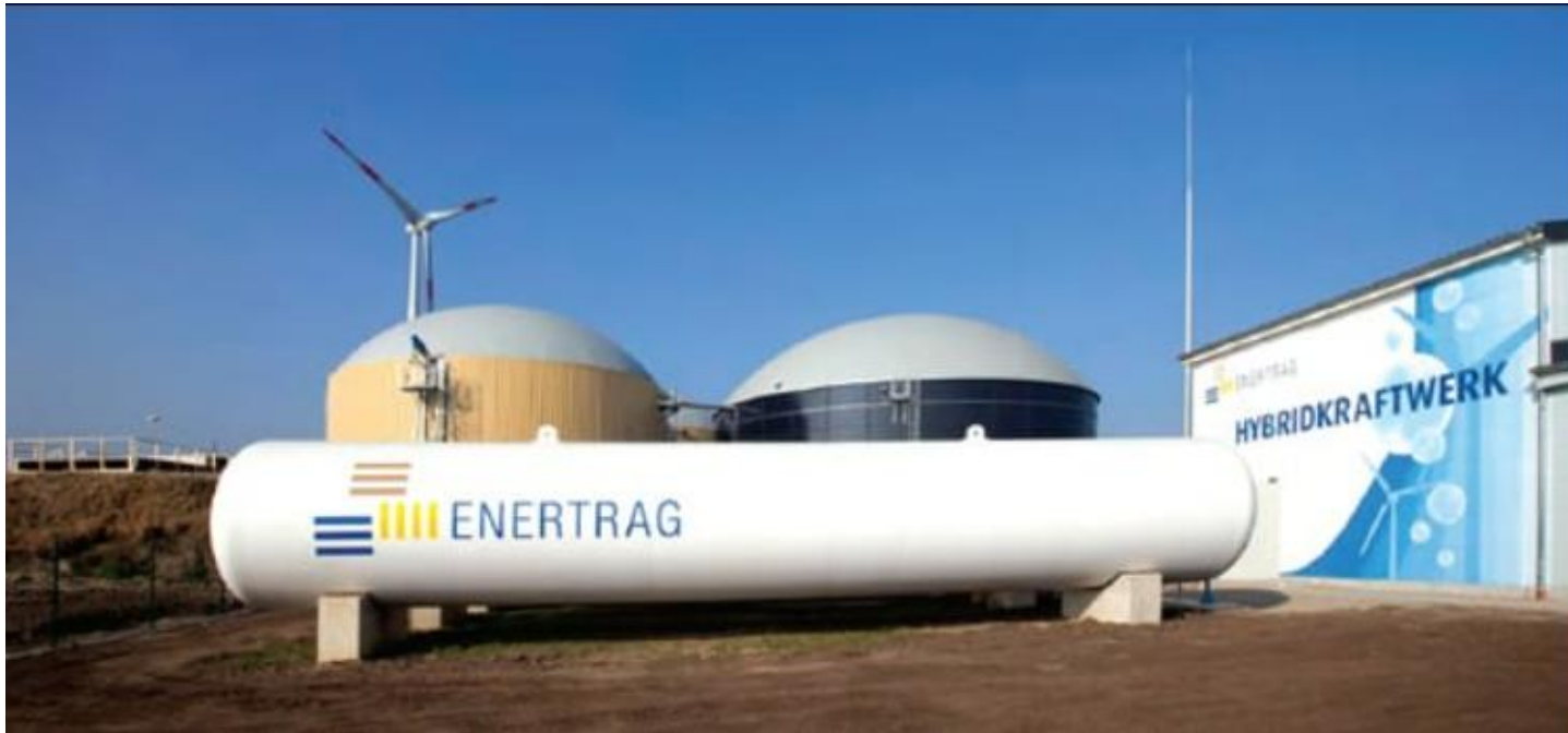
Figure 17: Compressed Hydrogen Storage – horizontal tank
