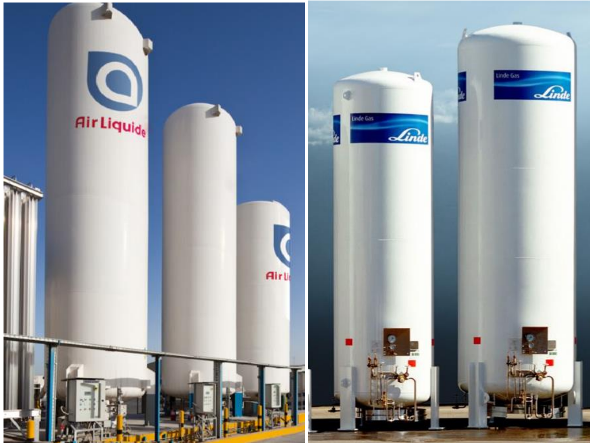
Figure 18: Cryogenic storage tanks – vertical tanks.
