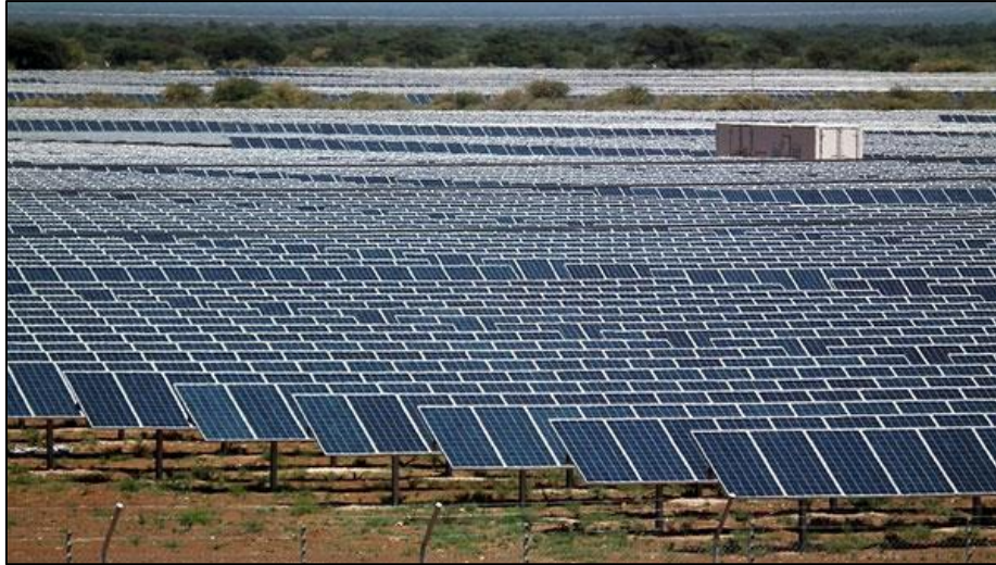
Figure 24: Kathu Solar Power Plant (photo courtesy of “visits to the park”), near Kathu, Northern Cape Province.
