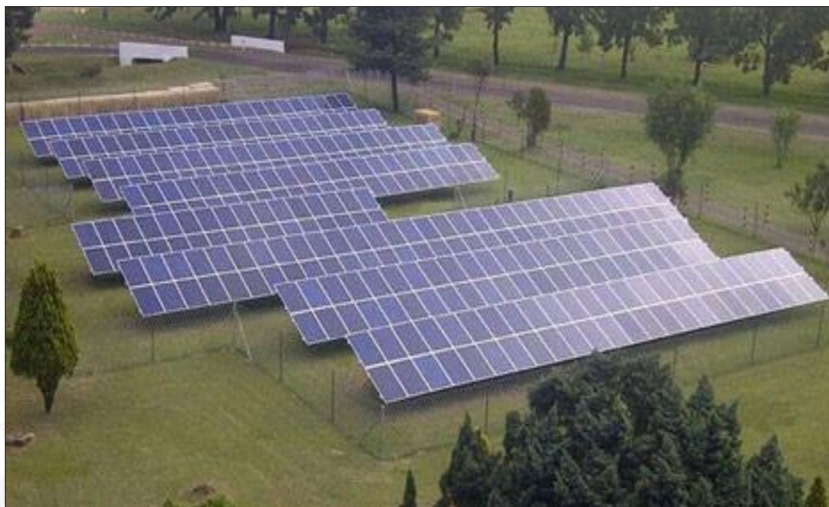
Figure 4: Solar PV Plant Array
