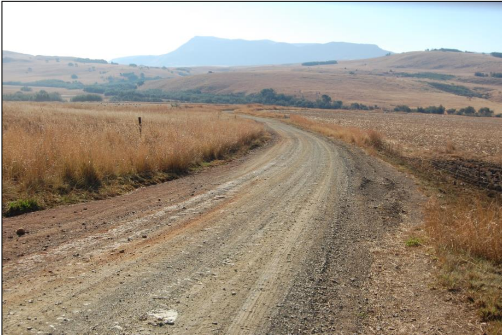
Plate 3 D699 – General Road Condition
