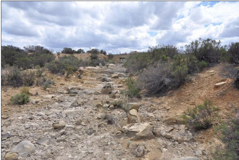
Plate 1: River bed erosion below an existing culvert.
