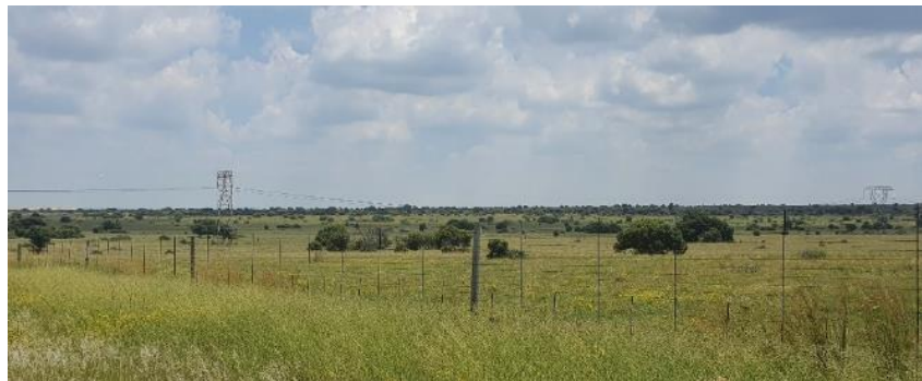
Figure 4-4: Hermes/Pluto 400 kV powerline
