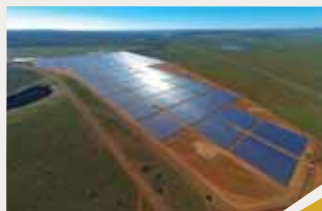
Structural, civil and electrical design review and site supervision on behalf of the owner's engineer for the Lesedi photovoltaic (PV) plant
