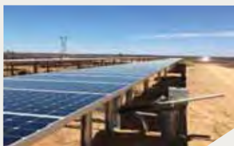
Prieska PV4 Facility - 81MW DC - Single-Axis Tracking PV
