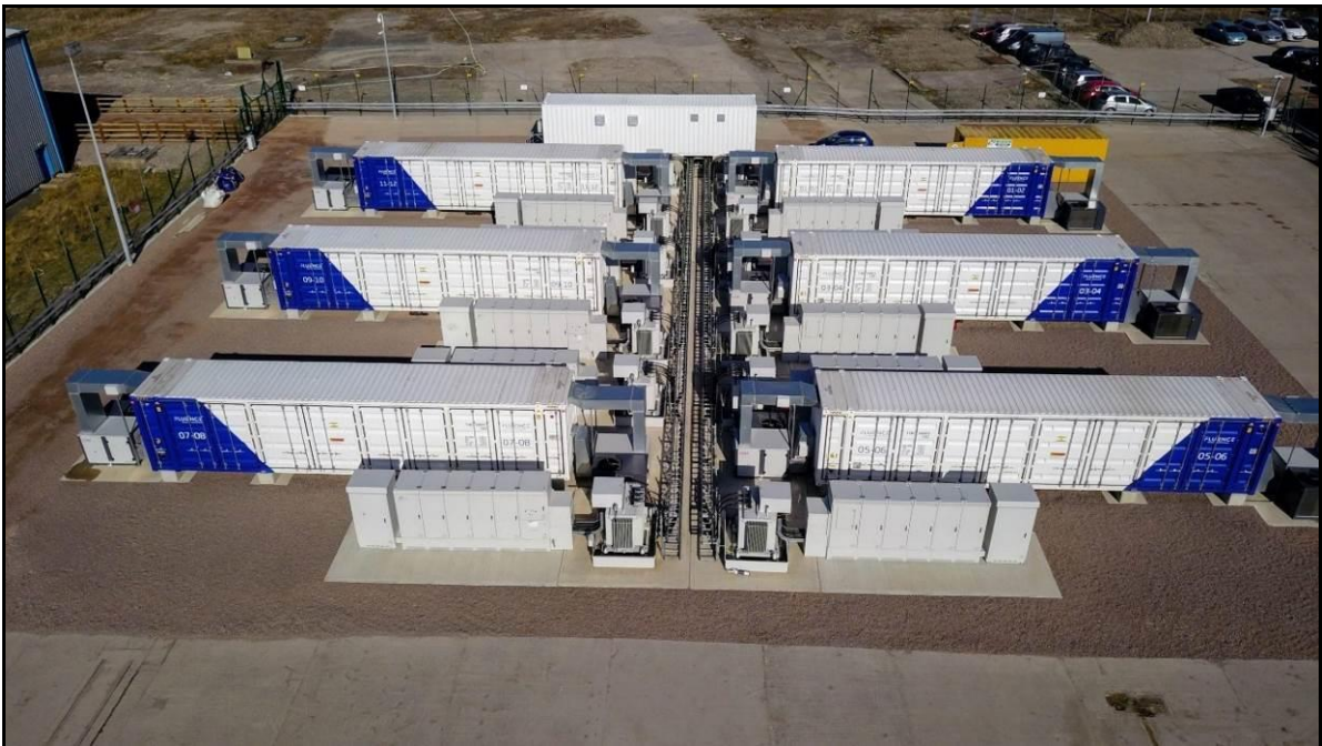
Photograph 1.2: Example of BESS located in storage containers
