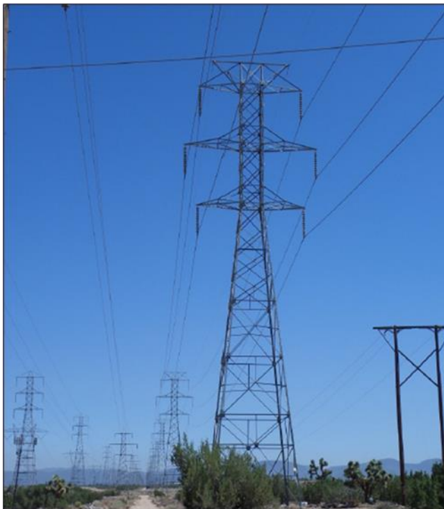
Figure 1-15: 132kV/275kV powerline double circuit suspension towers
